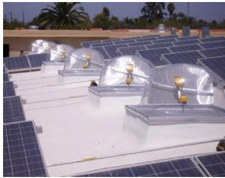
Ciralight Suntracker 400s on the roof of San Diego Gas & Electric's Innovation Center
