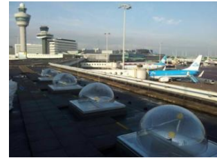
SunTracker 400's installed at Amsterdam International Airport
