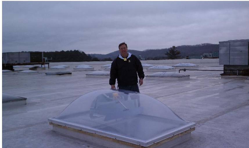
Jim Witt, of The Energy Solution Group, with a recently installed SunTracker 800 at GE
